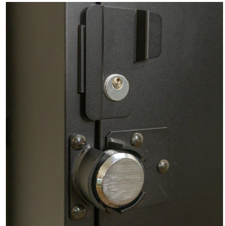
Fig. 14 – Single puck lock on cabinet door
